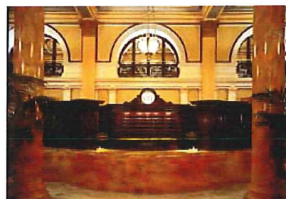
After rehabilitation, this severely deteriorated space was returned to its original elegance. Plaster was repaired and repainted; scagliola columns were restored to match marble; and missing decorative metalwork was re-installed in front of the windows. Photo: Carol M. Highsmith.
